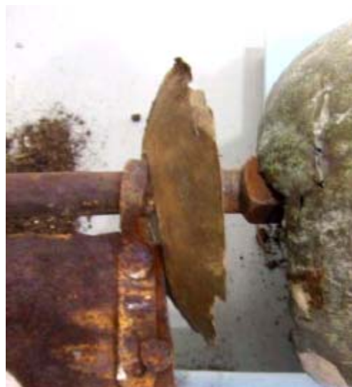
Figure 4: Deformation and iron corrosion products on the iron structure of the Yamur before restoration. Image: Eugenio Fernández Ruiz (IAPH)
